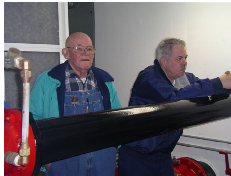
Commissioners John Thompson from WD 125 (left) and Russ Pritchard from WD 20 (right) inspect the new security improvements at the reservoir
